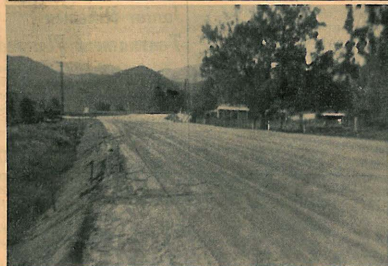
County Road Crews have been busy the past two weeks eliminating the sharp dangerous corner at the intersection of Harbison Canyon and Dehesa Road. Nearby residents have already noticed the change in traffic flow on busy weekends. The pictured corner has been the scene of several fatal accidents in the past few years.
